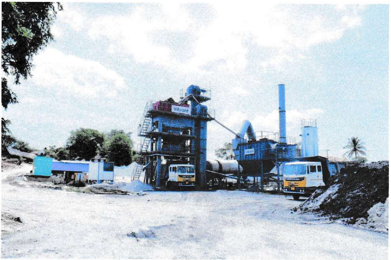
HSR Infra Projects Batch Mix Plant, Gudlanayanapalli Village, Kuppam, A.P
